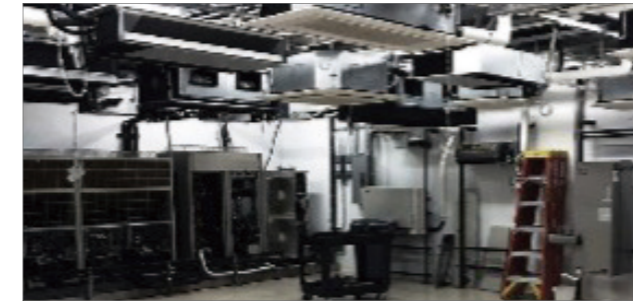
LG Air Conditioning Academy
